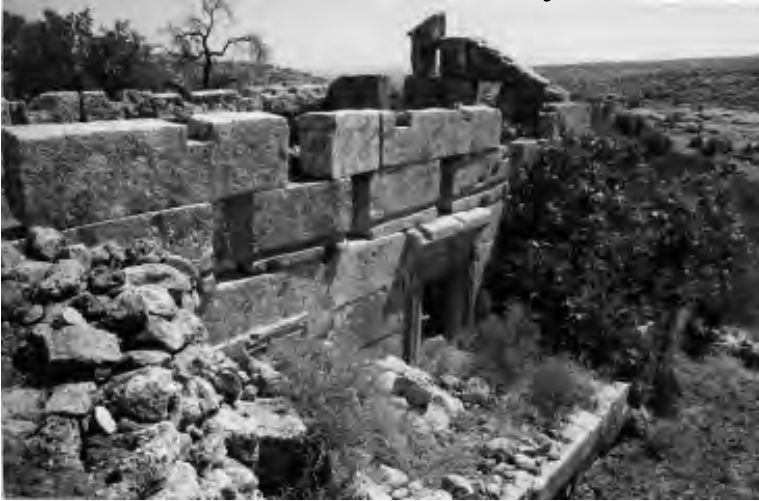
Figure 28.2a Church of Ma'ramaya, southern façade and baptistry at the eastern extremity of the portico
